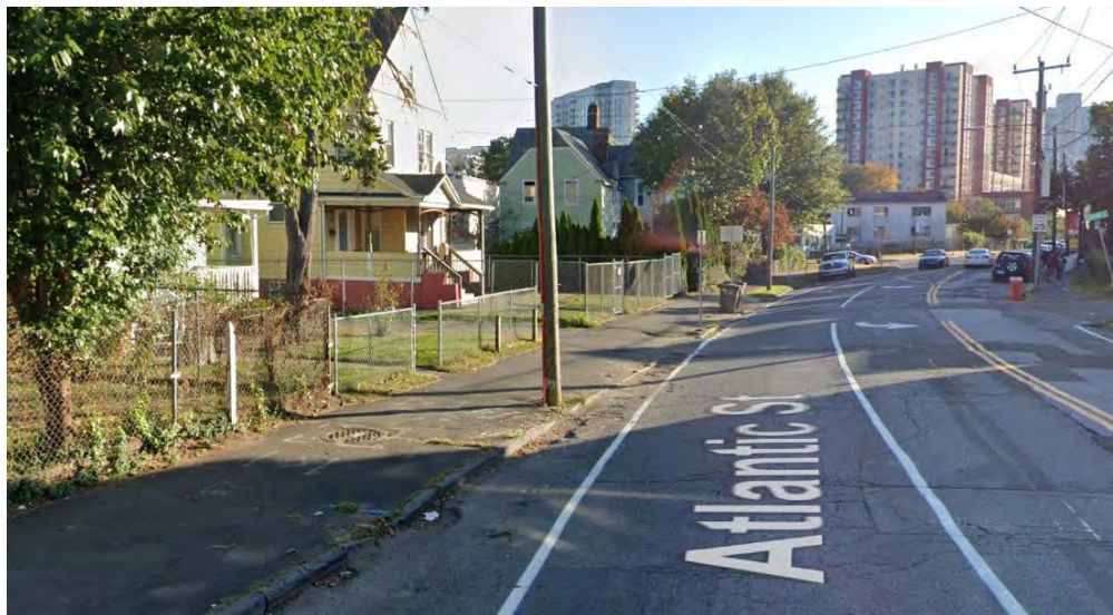
Exhibit 8 Uneven asphalt sidewalks on Atlantic Street
