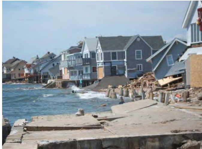
Hurricane Damage on the Connecticut Coast (Photo credit: CT DEEP)
